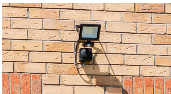
Rear security light with PIR
